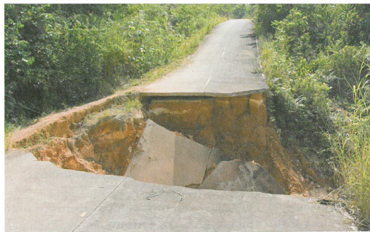
FIGURE 1.16 Human modification of Earth includes severe soil erosion. This asphalt road in Koh Chang, Thailand, has collapsed due to soil erosion. (Oleg D./Shutterstock.)
